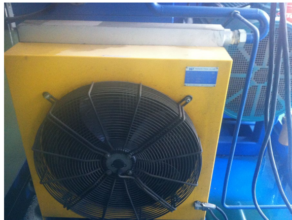
Fig. 4 The radiator in the cooling system
